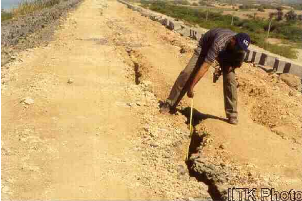
( Damage to Earthen Bund)
