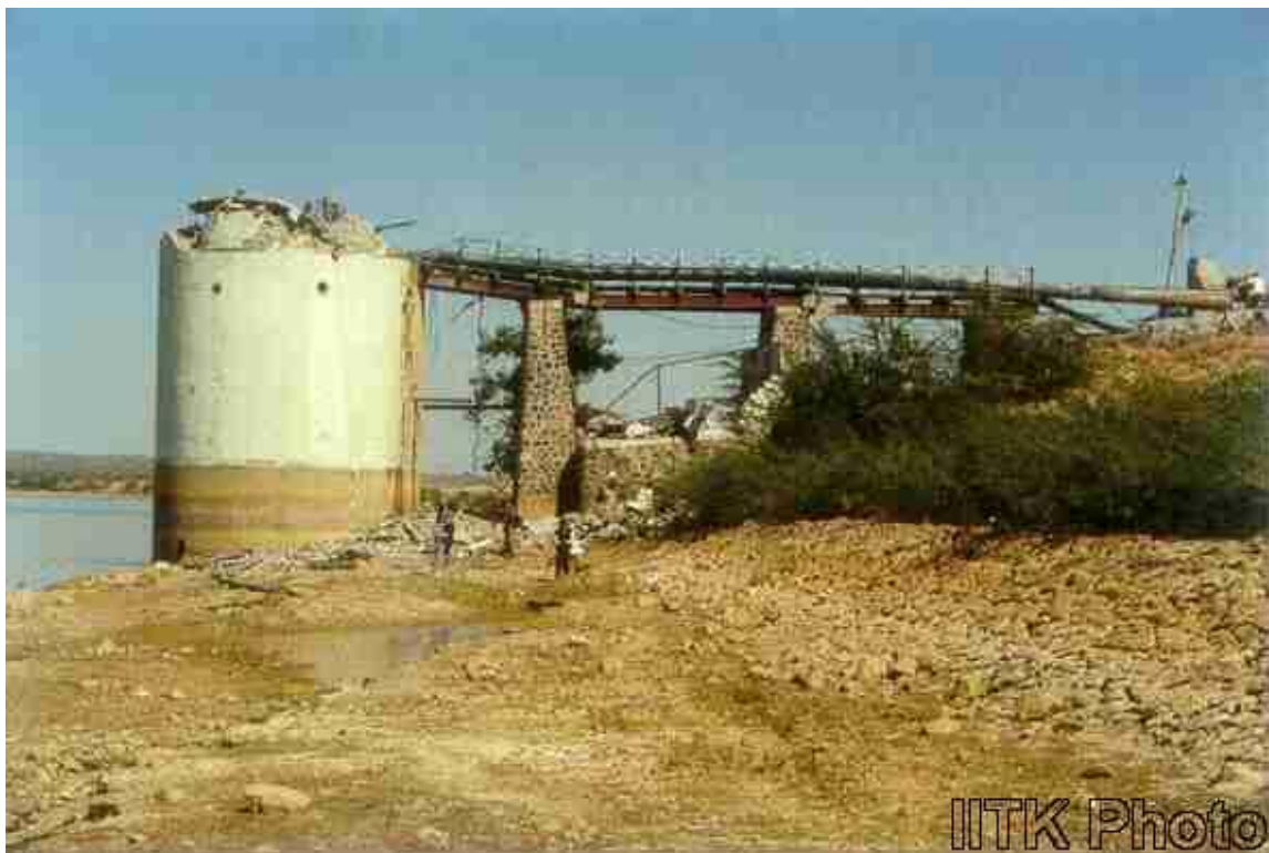
( Damage to Old Intake Structure and approach bridge)
